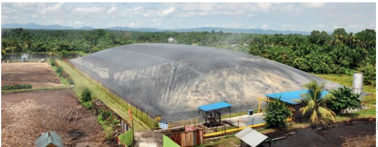
Pengembangan PLTBg berbasis POME. Biogas power plant based on POME.
